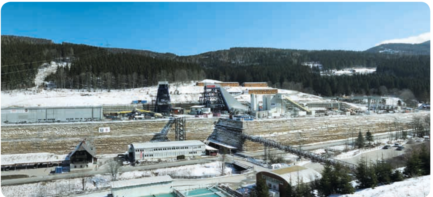
The tunnel excavation is taking place in two directions from the Fröschnitzgraben access shaft south of Steinhaus am Semmering. The first trains will be travelling through the Semmering base tunnel from 2026.
