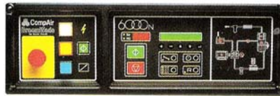
View of computerised control panel
